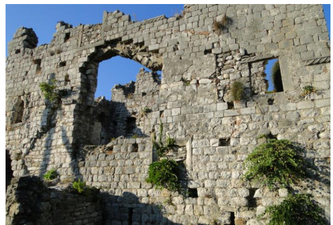
Figure 15: Example of destructive effects occurred on the ancient historical centre of Bar during the 29 May 1979 earthquake
